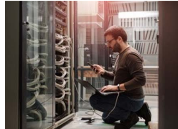
Building Systems & Controls
